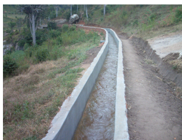
Canal diverting water to run the turbine
